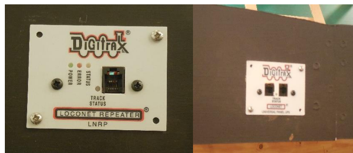
Pic 2: Digitrax Loconet panel modules were installed around the layout.
