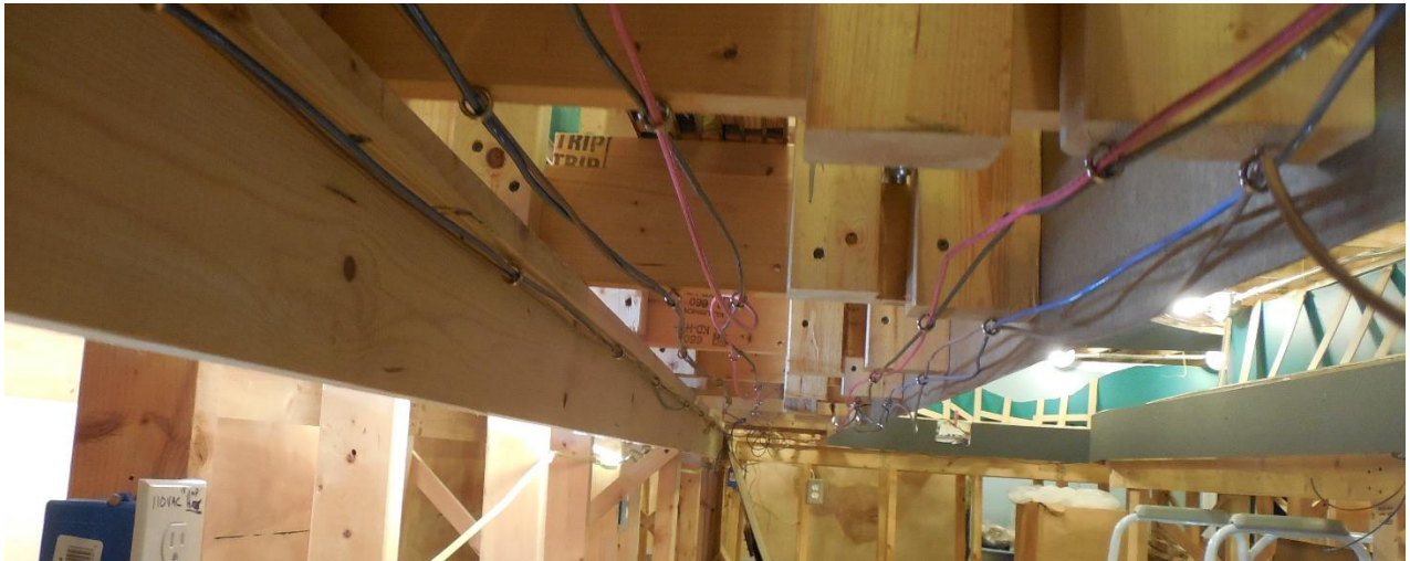
Pic 3: Screw eyes with a 3/8" opening are inserted into benchwork to provide support for the bus wires running to each of the planned 34 districts.
