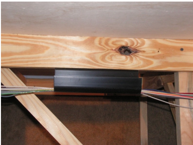
Fig.1 Cable tray under Black Cat Sta. layout.
